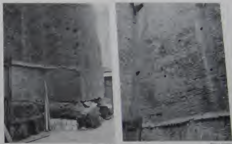
Fig. 10. View of terrace wall and substructure. Fig. 11. Detail of window opening in brick wall, showing arch and brickwork.
